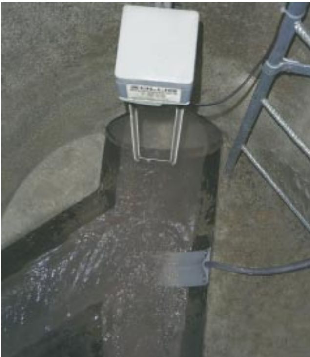
Inspection chamber with venturi nozzle and ultrasonic reference probe
