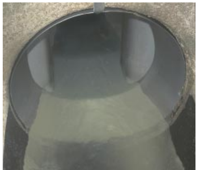
Venturi nozzle installed in pipe
